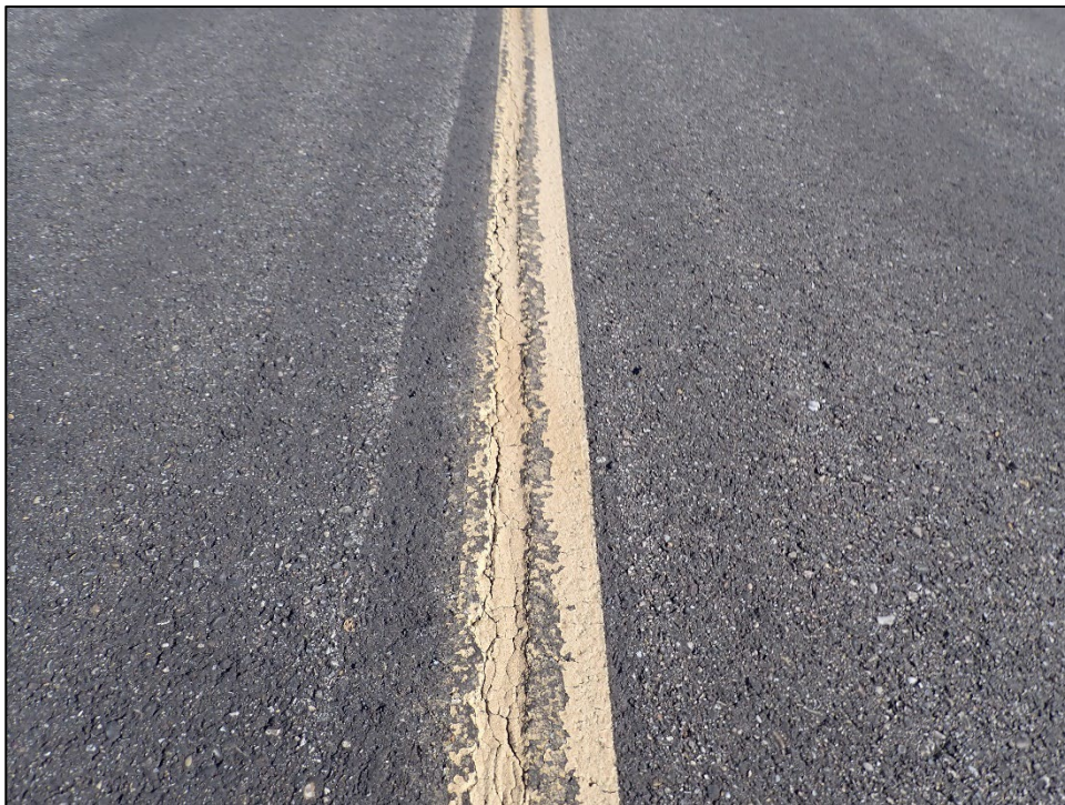
TW-02-01: L&T Cracking
